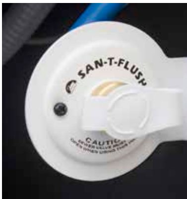
Typical black tank flush
