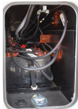
Typical Class A motorhome auxiliary battery compartment
