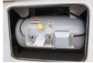
Typical propane gas tank
