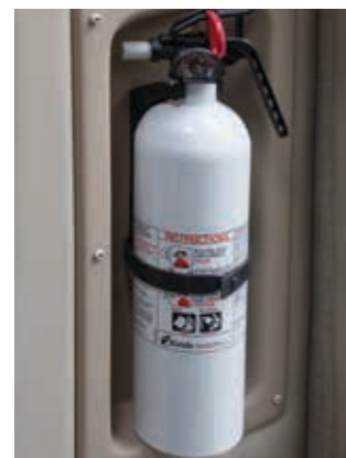
Typical Class B-C fire extinguisher
