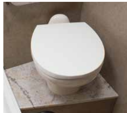
Typical motorhome toilet installation
