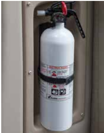
Typical Class B-C fire extinguisher
