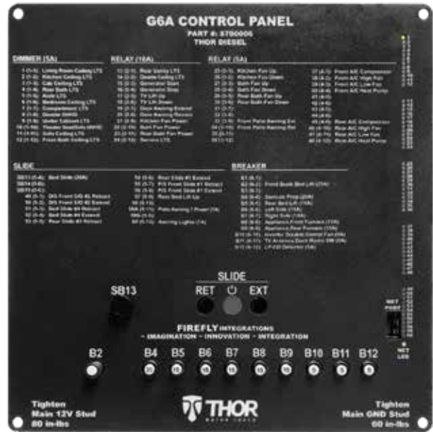
Typical 12 volt circuit breaker panel for Firefly multiplex system
