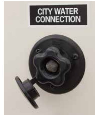
Typical city water fill connection
