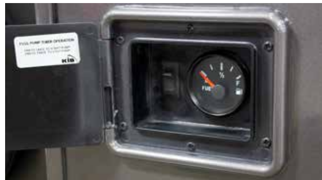
Fuel Pump Switch and Fuel Gauge for Fuel Transfer System
