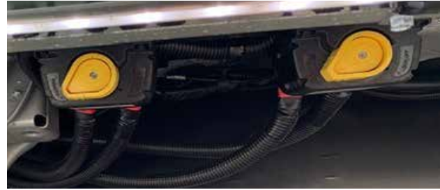
Safety Relays for the Li-ion Battery System
