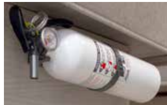
Typical Class B-C fire extinguisher
