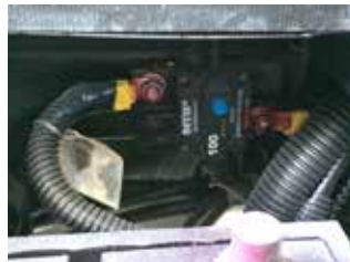
Typical Inverter Circuit Breaker
