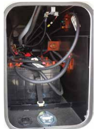
Typical Class A motorhome auxiliary battery compartment
