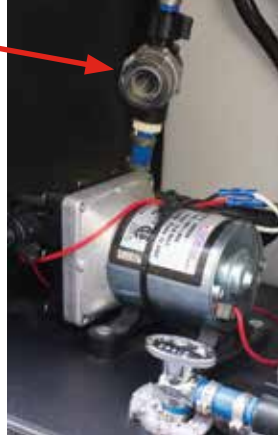
Water pump strainer
