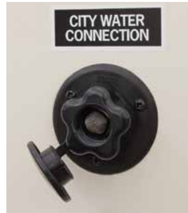
Typical city water fill connection
