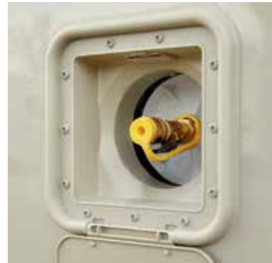
Typical external propane hook-up
